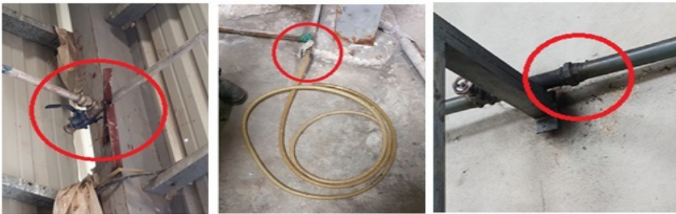
Figure 9. Photographic image of leakage points
